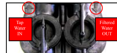
Inlet and Outlet Bypass Valves Open
