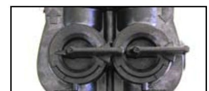
Inlet & Outlet Bypass Valves Closed
